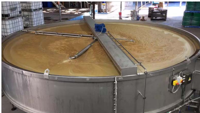
Continuous separation basin with rotating suction heads to remove floats – new installation (2017)
