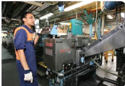
The Revesby facility incorporates 12 bodymaker and trimming pairs. Control panels on each incorporate operator interfaces wired to distributed I/O, plus a InView message display.
